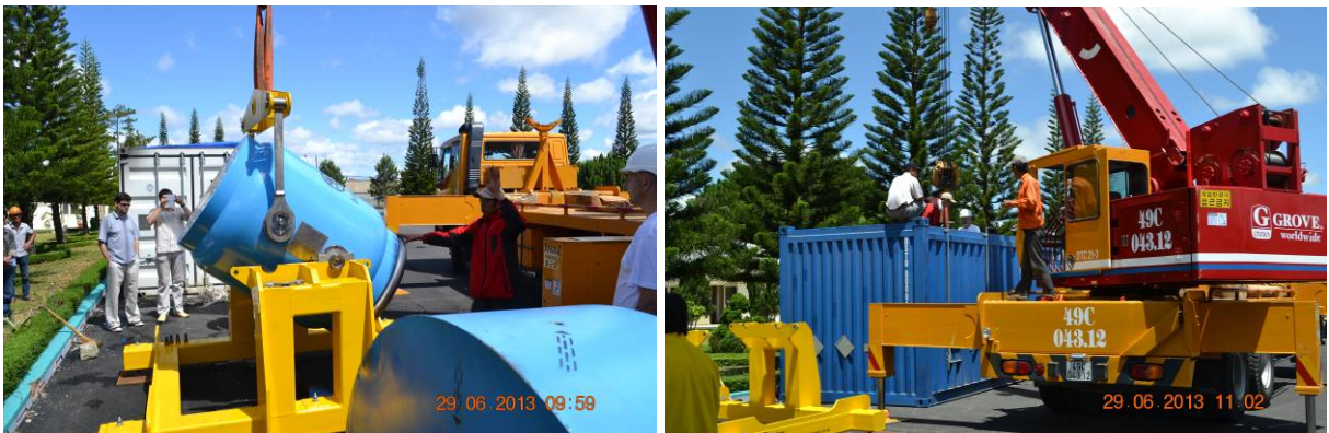
Fig. 7. Installing the SKODA VPVR/M cask in the tilter, loading into ISO container
