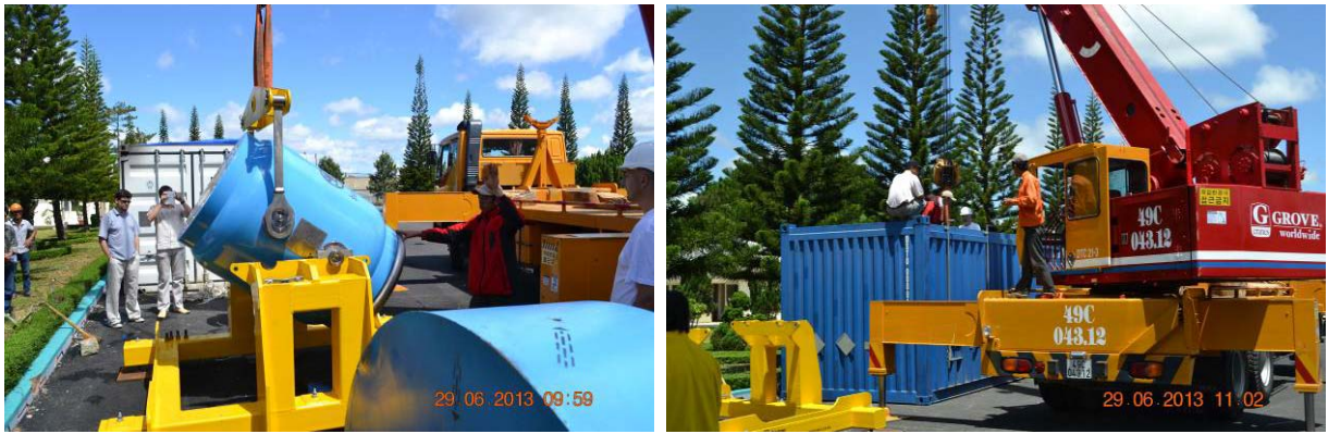
Fig. 7. Installing the SKODA VPVR/M cask in the filter, loading into ISO container
