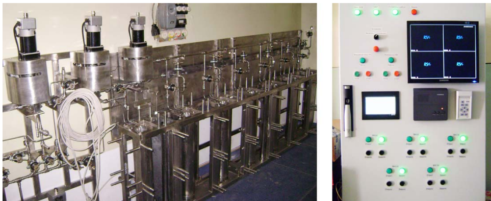
Fig. 1. Half-mounted equipment for LSNF discharge and temporary storage in the reactor hall
